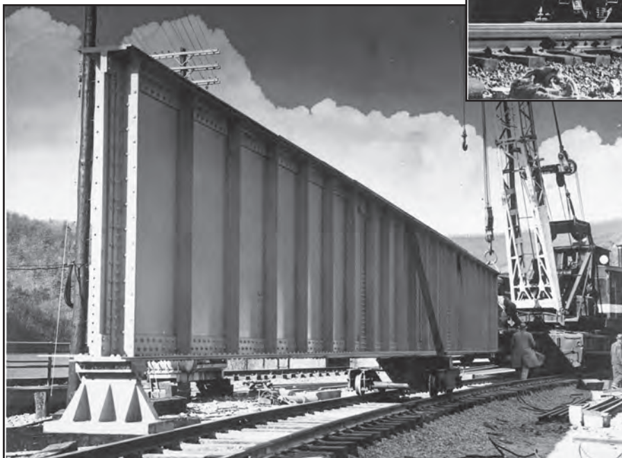
Side plate-girder assembly sitting on a pedestal with pin-bearing in the foreground, and a four-wheel dolly or cart in the back, controlled by a crane. You can see the pre-drilled holes above the bottom angle-channel for attaching the deck assemblies. (C&OHS Collection, CSPR 10117-6)
