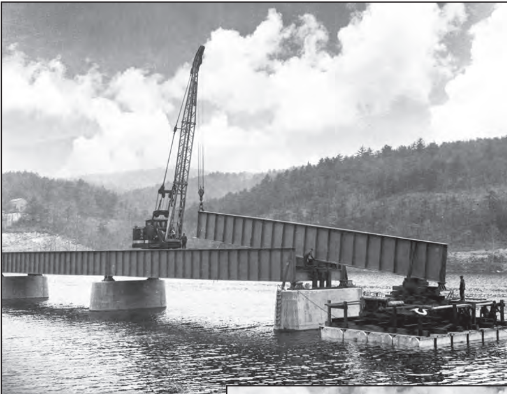
Gray primed side-plate-girder being passed through a complete span riding on pontoon falsework for attachment to the next pier, to be set on the pier's cap fixtures. (C&OHS Collection, CSPR 10117-3)
